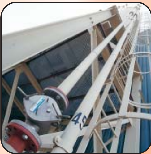
Magnetic filter in pneumatic transport pipeline for filling storehouses like e.g. for sugar, soy, flour, plastics, spices etc.
