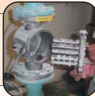
Industrial filter in a pneumatic conveying system, used for deferrising flour.
